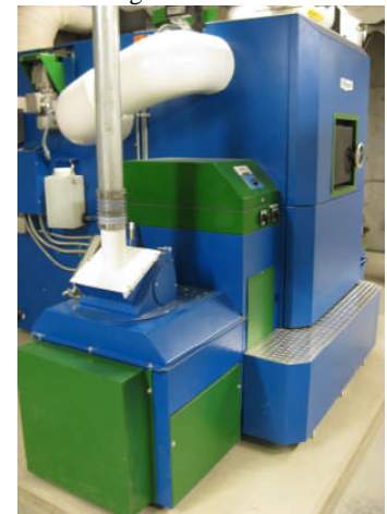
Fig. 3 Side of Boiler showing vertical pellet auger delivery tube
